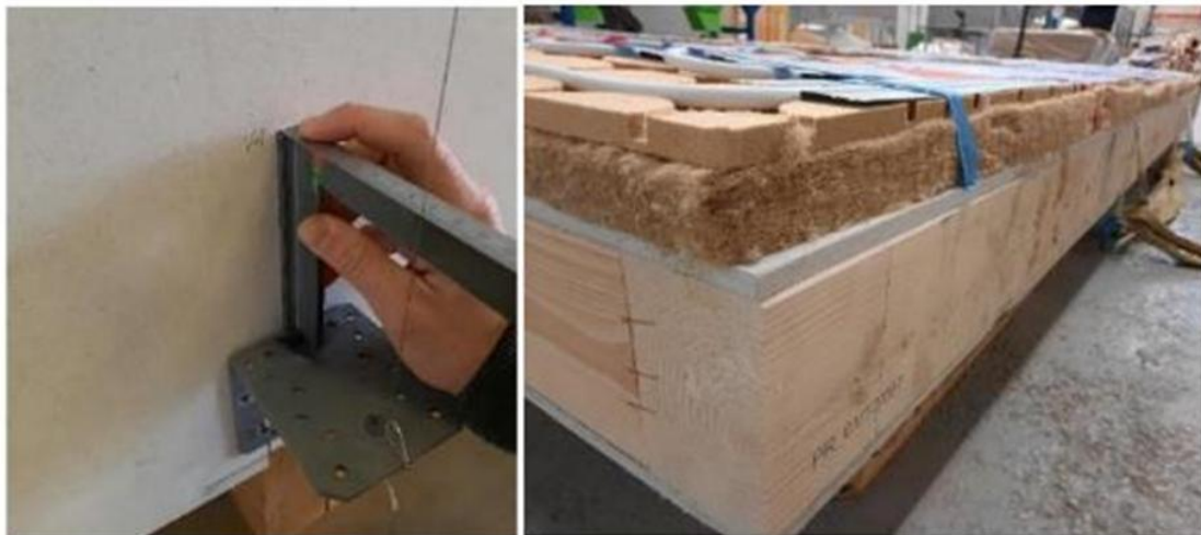
FIGURE 29: THE DISTANCE BETWEEN THE FAÇADE ELEMENT WAS MEASURED WITH A CARPENTER ANGLE TO INCREASE THE ACCURACY OF THE MEASURED POINTS. THE MEASUREMENT IS NECESSARY AS THE FLEXIBLE LAYER ON THE RIGHT GETS COMPRESSED WHEN THE MODULE IS INSTALLED. THIS RESULTS IN A HIGH FORCE ON THE COMPLETE MODULE THAT MAY CAN DEFORM IT.
