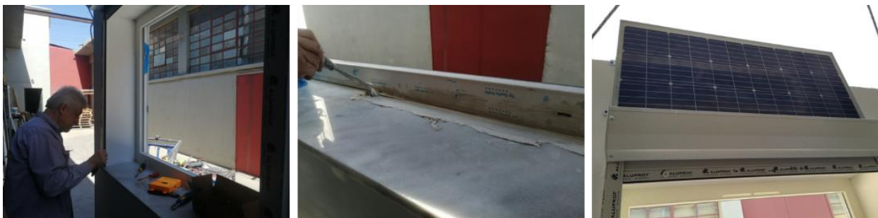
FIGURE 3: (LEFT): LOCAL REPAIRS ON THE CORNER BEAD, (MIDDLE): SEALANT REPAIRS, (RIGHT): PV RE-ALIGNMENT.
