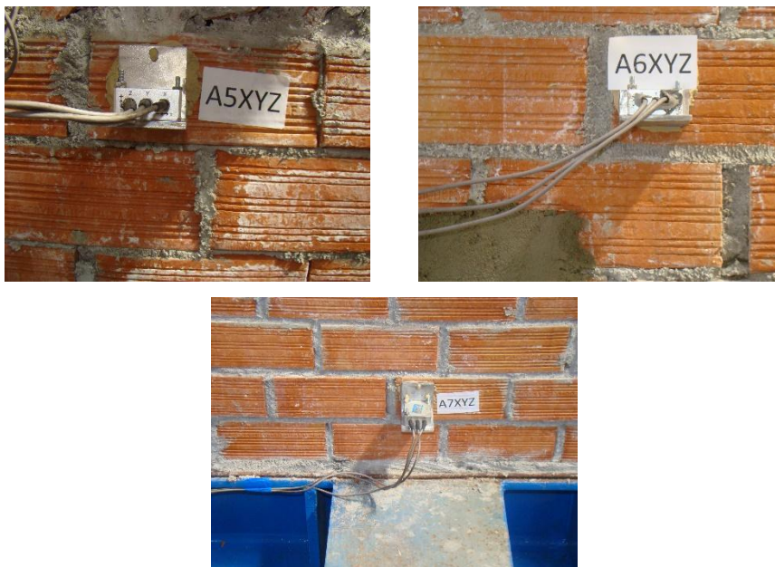
FIGURE 109: INSTRUMENTATION SET-UP: ACCELEROMETERS PLACED AT MEASUREMENT POINTS A5, A6 AND A7 (BRICK WALL)
