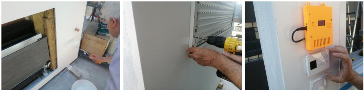
FIGURE 2: (LEFT): RECOATING DAMAGED AREA, (MIDDLE): REPLACING DEFECTIVE SCREWS, (RIGHT): ALIGNMENT FAN-COIL'S CONTROL UNIT.
