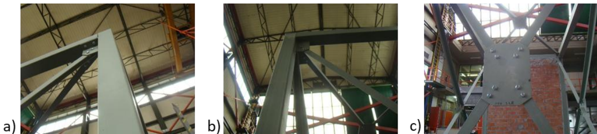
FIGURE 13: A) BEAM TO COLUMN BOLTED CONNECTION; B): WELDED BEAM TO COLUMN JOINTS AND C) MID-HEIGHT CONNECTION OF X-BRACES.
