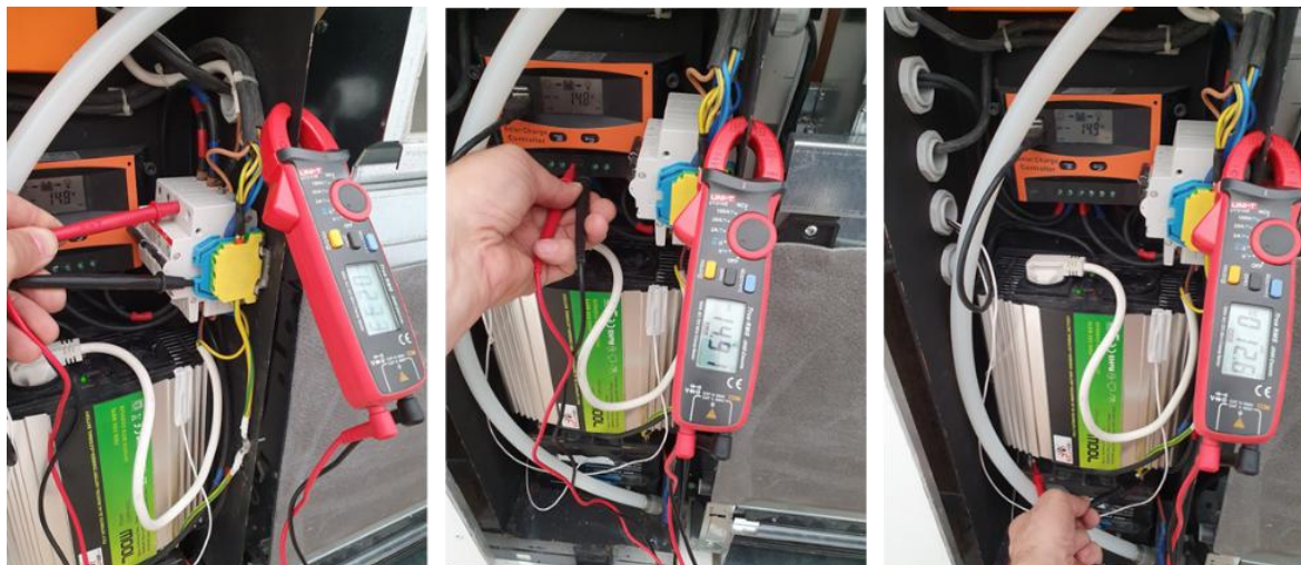
FIGURE 7: (LEFT) LINE CONTINUITY TEST, (MIDDLE): CHARGER INVERTER TEST, (RIGHT): INVERTER VOLTAGE TESTING
