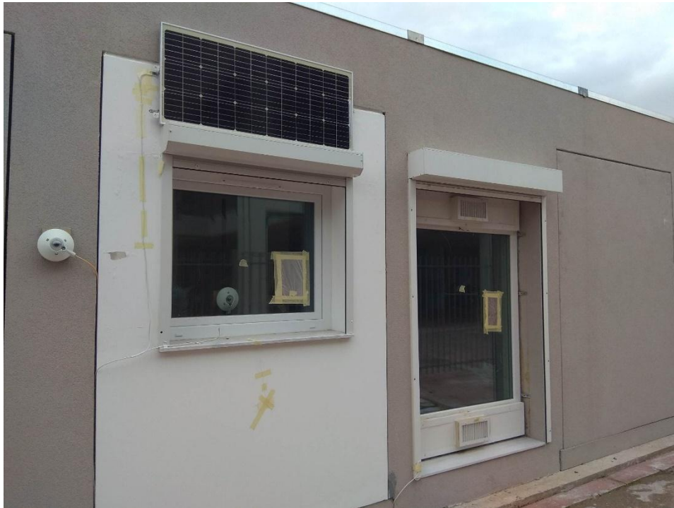
FIGURE 85: THE INSTALLED SMARTWALL AND SMART WINDOW PROTOTYPES AT NTUA LIVING-LAB.
