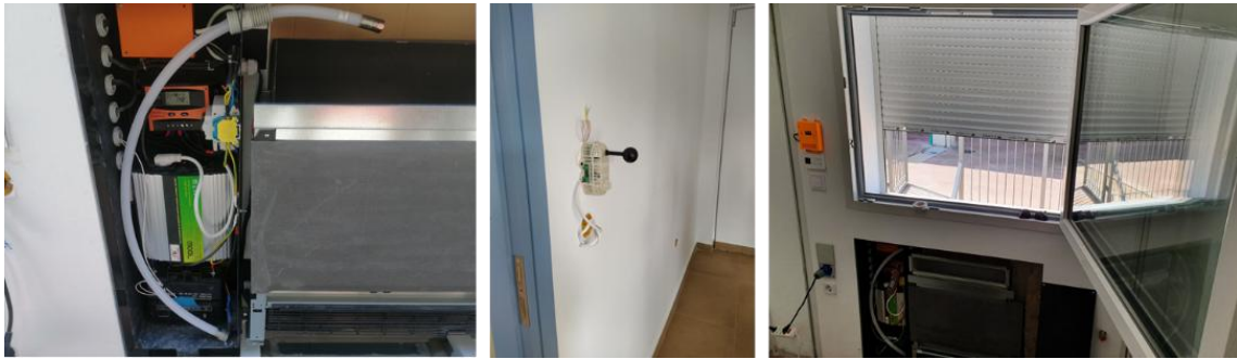
FIGURE 9: (LEFT) TOOLBOX TESTING, (MIDDLE) SENSOR TESTING, (RIGHT): BLIND ROLLERS TESTING.
