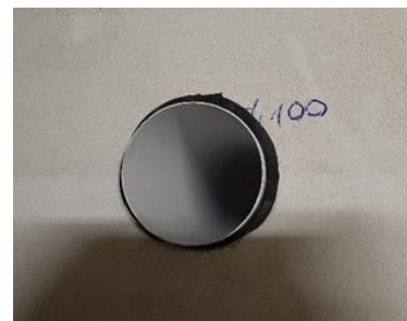
FIGURE 51: DETAIL OF THE SUPPLY AIR OUTLET TO THE OPPOSITE SIDE OF THE DIVIDING WALL (FACING THE RECEIVING ROOM)
