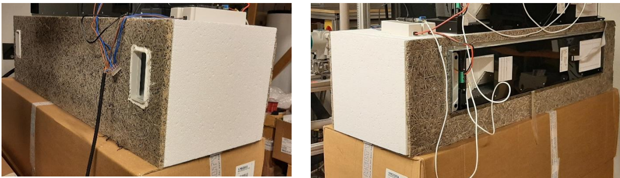
FIGURE 19 : VENTILATION UNIT HELTY FLOW 70 IN INSTALLATION BOX (EXTERIOR SIDE – LEFT PICTURE; INTERIOR SIDE WITHOUT PANEL– RIGHT PICTURE)
