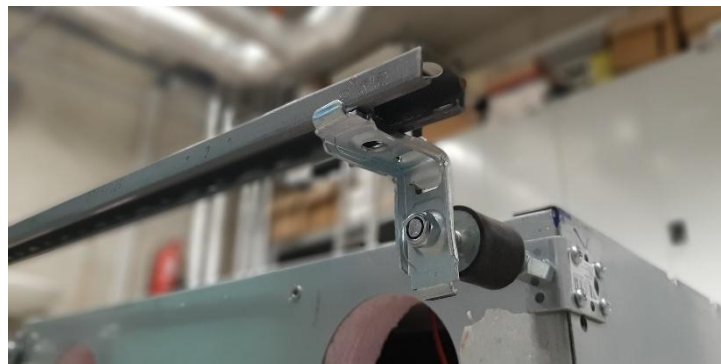
FIGURE 51: ANCHOR OF VENTILATION UNIT WITH SILENBLOCK
