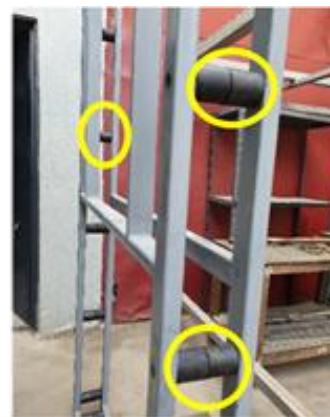
FIGURE 61: RUBBER SPACERS BETWEEN PANEL’S METAL FRAMES
