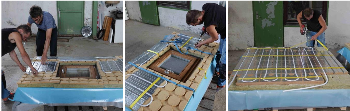
FIGURE 36: MANUFACTURING STAGE #4 (E/M COMPONENTS INSTALLATION) – HEATING LAYER WITH INSULATION AND HEATING PIPES
