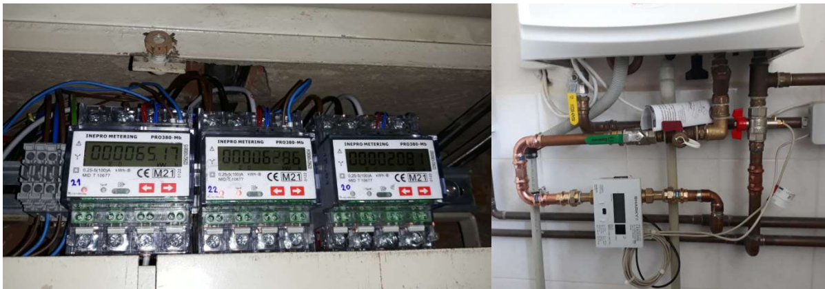
Figure 4 Smart energy meters for electric consumption measurement and calorimeter for heat demand
